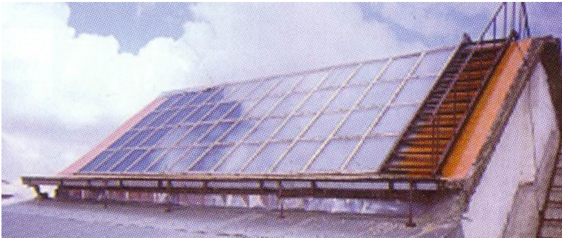
Fig. 6.7 Photograph of solar air heating system at the HP State Co-operative Bank, Shimla [2]
